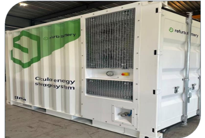
Battery Energy Storage
